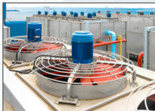
Fan and water pump
